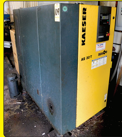
Kaeser Air Compressor, 1 of 2
