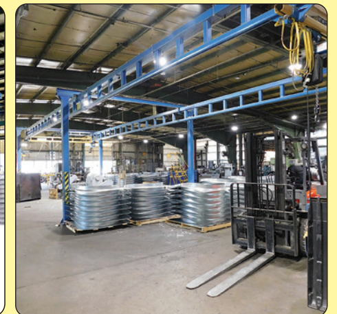
Gorbel 1 Ton Free Standing Crane (1 of 3)
