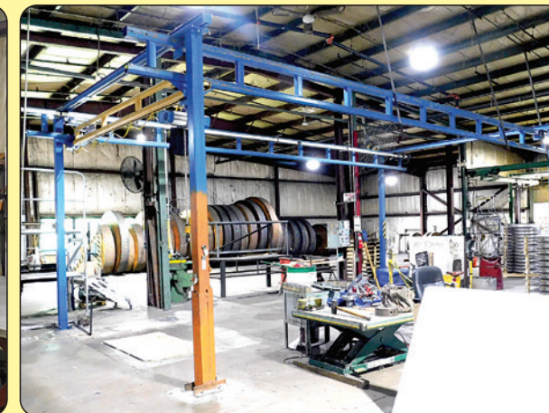
Gorbel 1 Ton Free Standing Crane (1 of 3)
